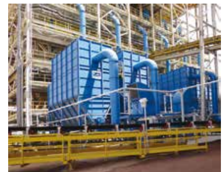
Bag Filter Systems in a Surface Mine, Mauretania
